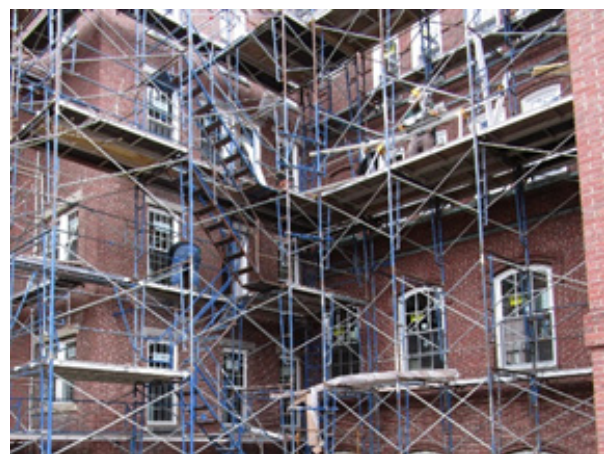
New windows approved by NH State Historic Preservation Office being installed at Main Building.
