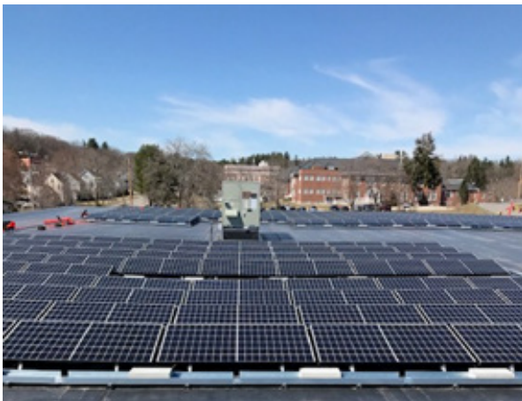
The Rooftop Solar PV system installed on the Records & Archives Building consists of 2 arrays with 240 solar modules totaling 73 kW DC.
